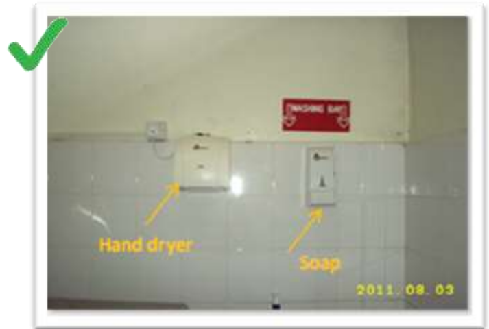
Figure 34: Adequate washing facilities must be provided
