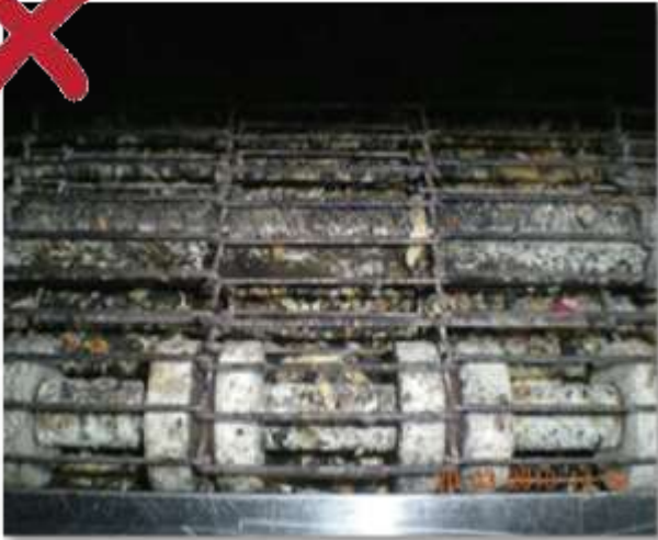
Figure 31: Conveyer belt design not suitable for cleaning since cannot be disassembled
