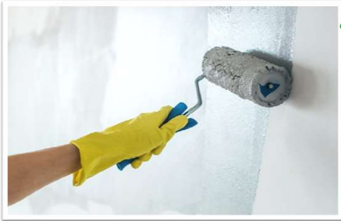
Figure 20: Surfaces of walls, partitions and floors should have smooth and impervious surface.
