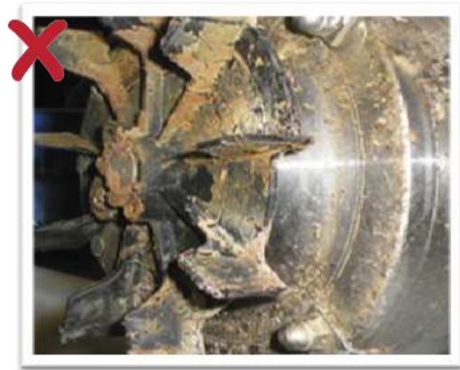
Figure 47: Rusted equipment with old sediments poses a food contamination hazard.
